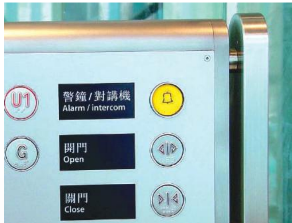
Figure 103: Lift Control Panel
